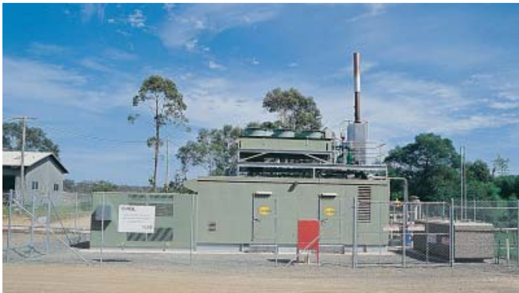
Landfill gas from the City’s West Nowra Landfill powers an on-site 1-Megawatt generating plant, producing electricity for Australia’s rapidly developing Green Energy’ program.
